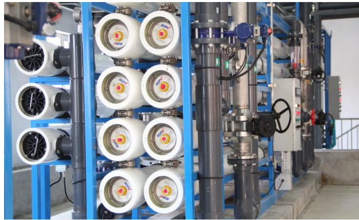
2,800 m 3 /d Seawater Desalination Project in Dalian
