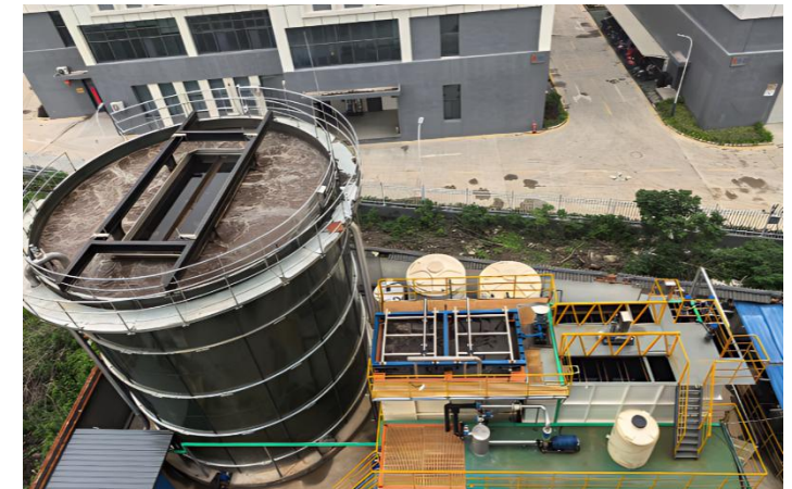
1,200 m 3 /d Printing & Dyeing Wastewater Treatment & Reuse Project in Changshu
