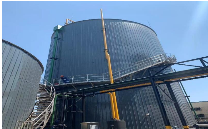
3,000 m 3 /d Soybean Wastewater Treatment Project in Zhejiang
