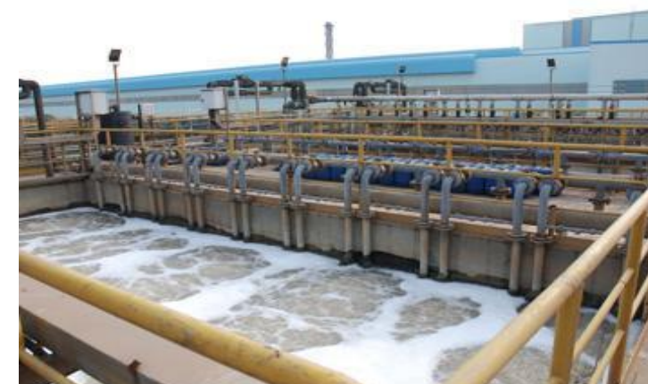
2,000 m 3 /d Steel Wastewater Reuse Project in Jiangsu
