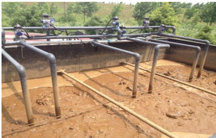
150 m 3 /d Incinerator leachate Treatment Project in Hubei
