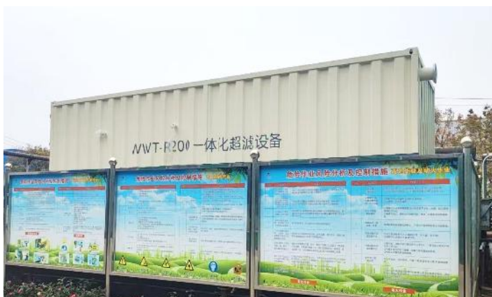
200 m 3 /d Kitchen Wastewater Treatment Project in Hubei
