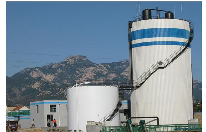
4,000 m 3 /d Beer Wastewater Treatment Project in Shandong
