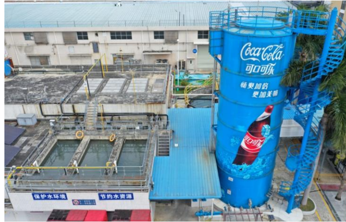
800 m 3 /d Food Wastewater Treatment Project in Guangxi
