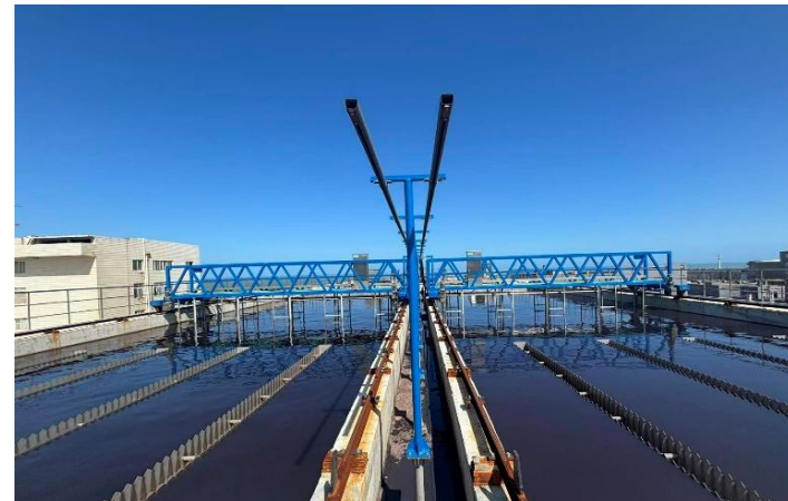
10,000 m 3 /d Printing & Dyeing Wastewater Treatment & Reuse Project in Fujian
