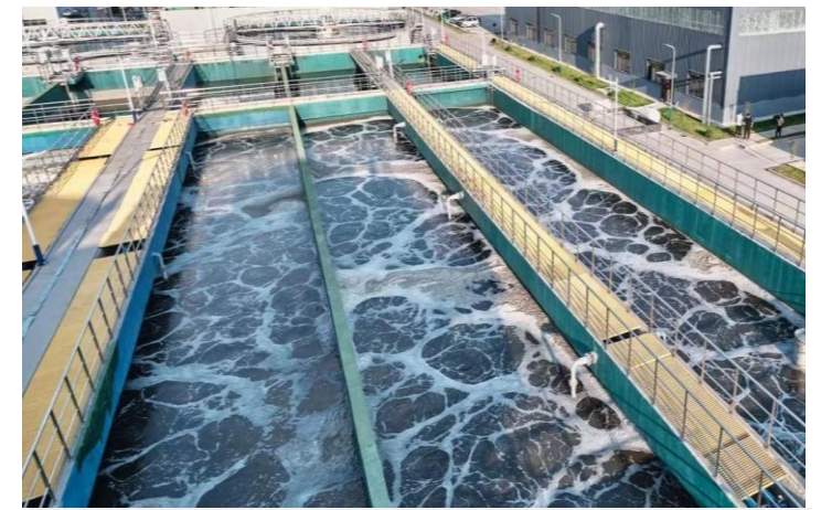
3,000 m 3 /d Steel Wastewater Treatment Project in Hubei
