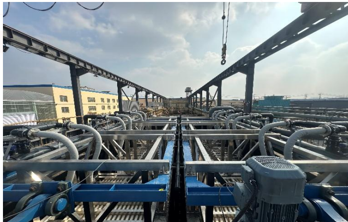
5,000 m 3 /d Printing & Dyeing Wastewater Reuse Project in Shandong
