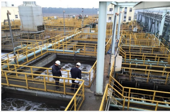
2,000 m 3 /d Steel Wastewater Treatment Project in Guangzhou
