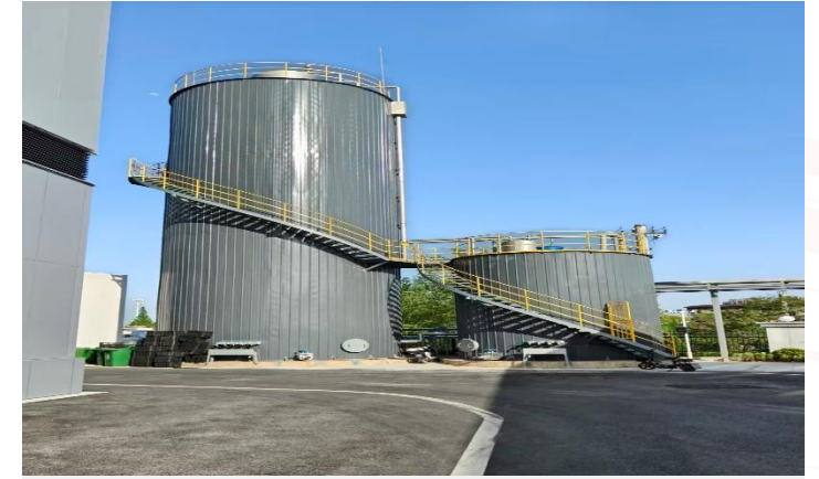
350 m 3 /d Food Wastewater Treatment Project in Anhui
