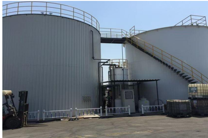
2,000 m 3 /d Food Wastewater Treatment Project in Anhui
