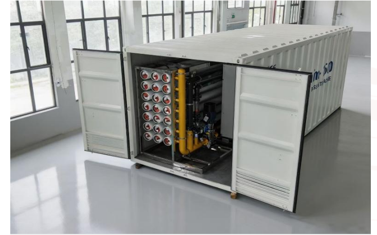
500 m 3 /d D&P Wastewater Reuse Project in Zhejiang
