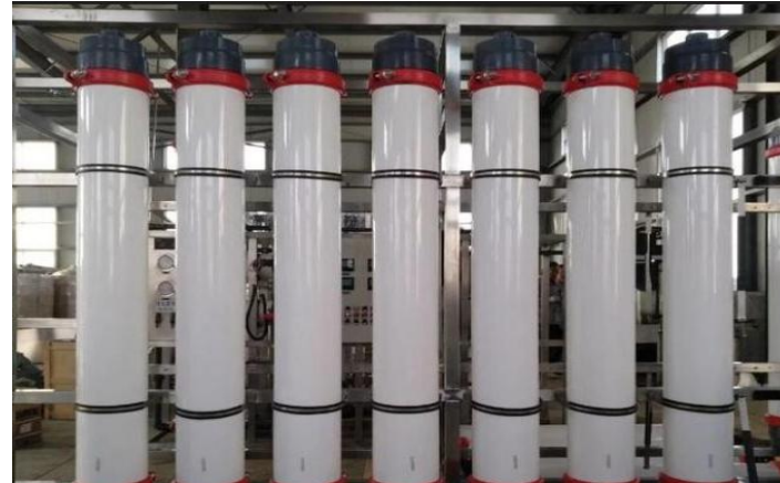
8,000 m 3 /d Municipal Sewage Reuse Project in Guangxi
