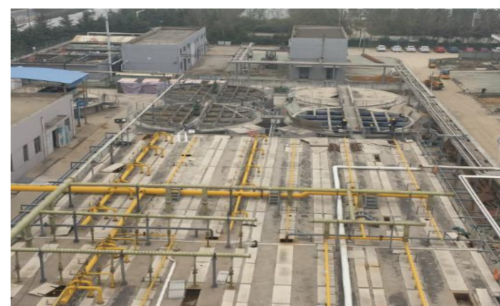
2,500 m 3 /d Pharmaceutical Wastewater Treatment Project in Lianyungang
