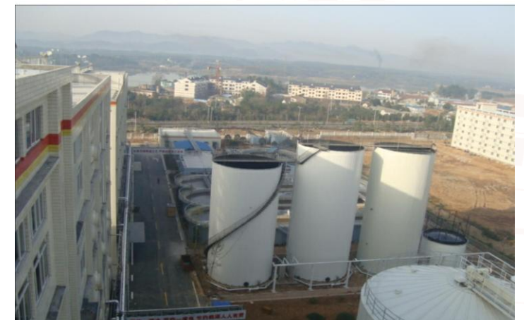
7000 m 3 /d Soybean Wastewater Treatment Project in Zhejiang
